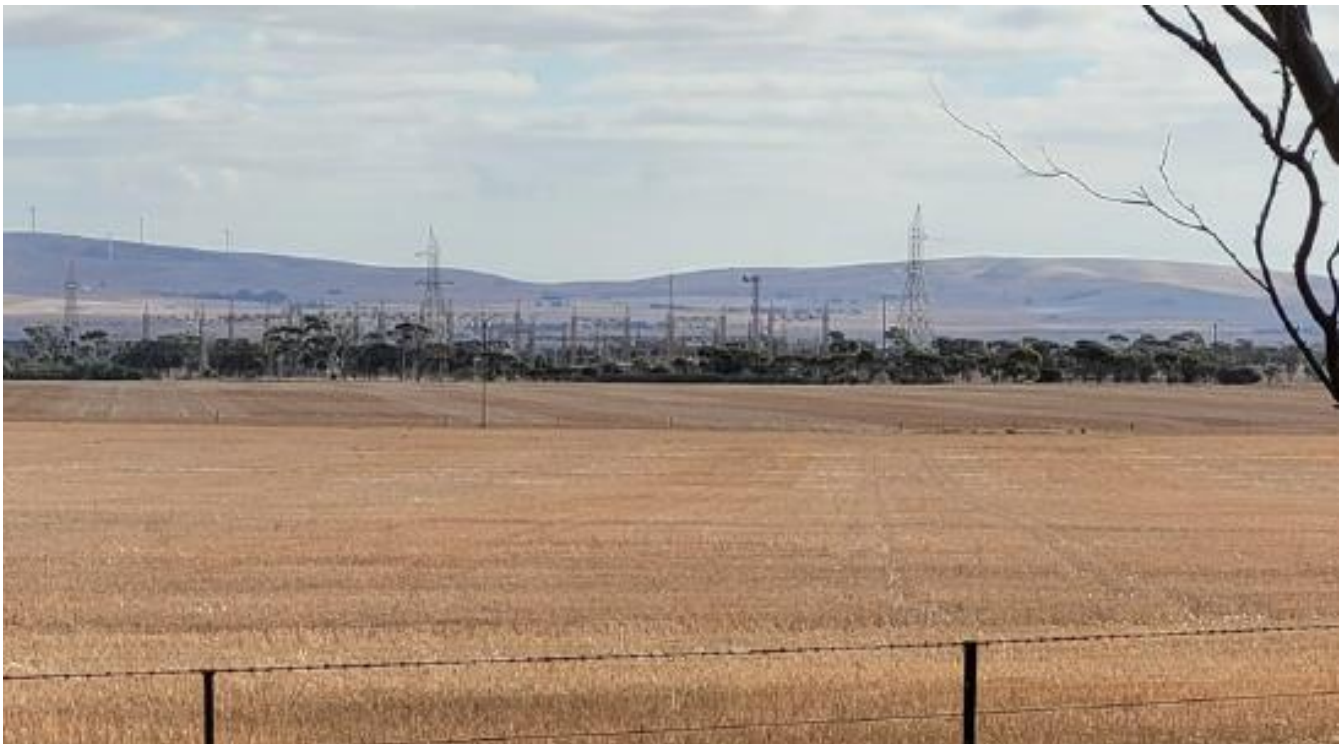
Figure 9: View of the Brinkworth Substation (with the Snowtown Wind Farm in the background)
