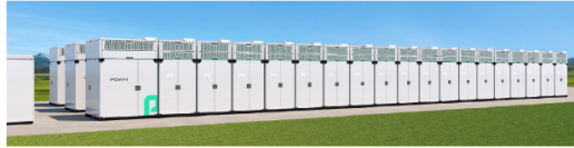
Example of a typical Battery Energy Storage System (BESS)
