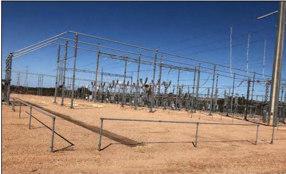
Figure 12e: Example substation
