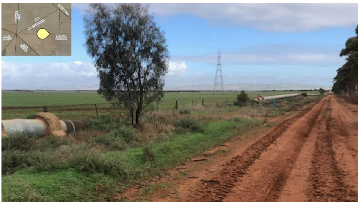
Figure 2.4: Boucaut School Road Water Main (looking west)
