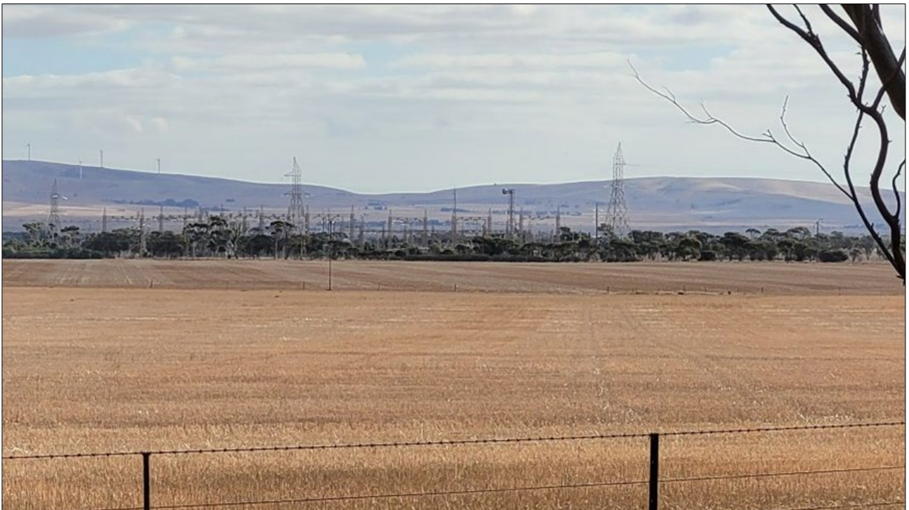
Figure 5. View of the Brinkworth substation and Snowtown Wind Farm in the background.
