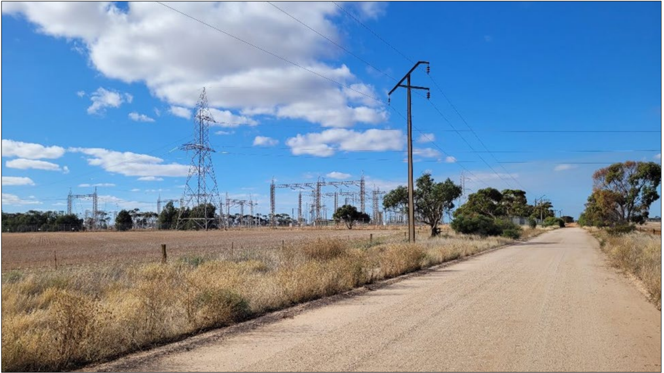
Figure 4. View of Brinkworth substation from Power Station Road.
