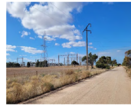
View of the existing Brinkworth substation looking north-east along Power Station Road
