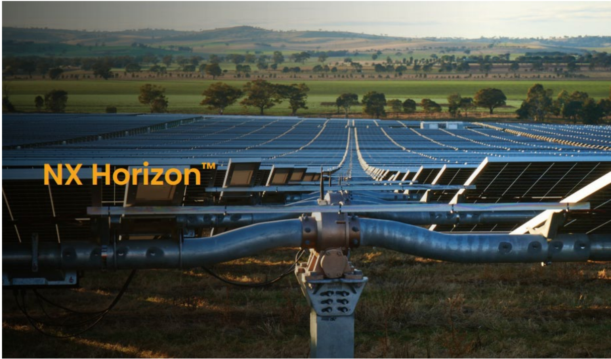
Figure 3-7 NEXTracker NX Horizon is the proposed mounting and tracking system for the Project solar panels
