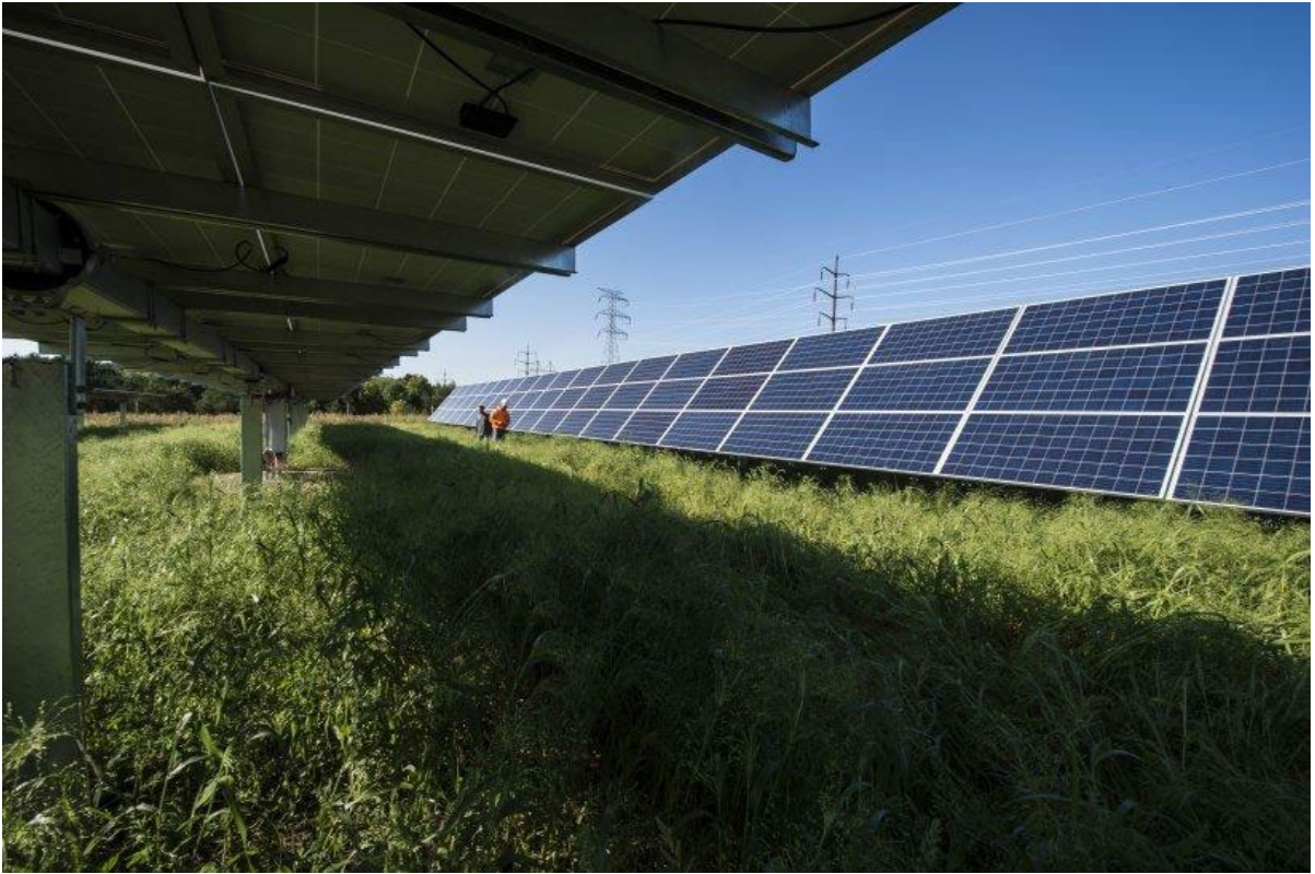
Figure 3-2 Typical single axis tracking solar array
