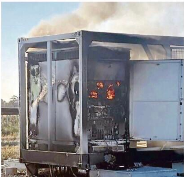
A transformer at a central Victorian solar farm caught fire late on Thursday. Picture CFA.
