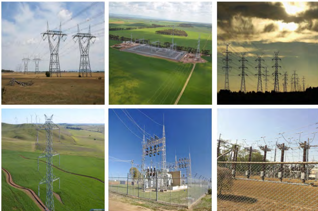
Figure 2-5: Existing Electrical Infrastructure in Australia
