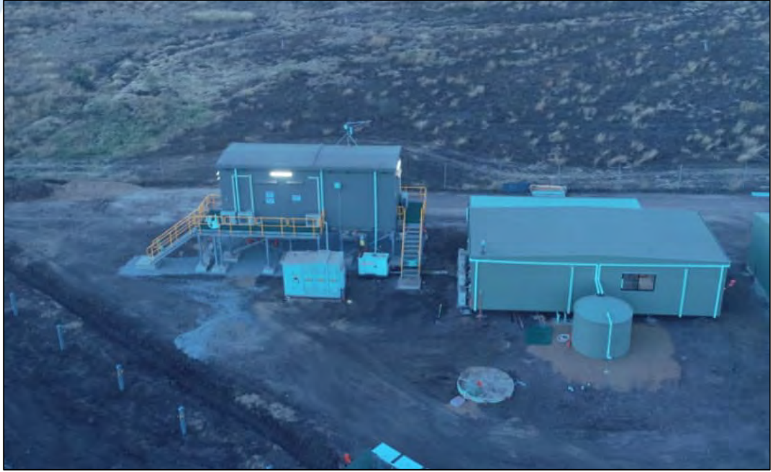
Figure 4-8: Example of a Typical Switch Room Alongside an O&M Building
