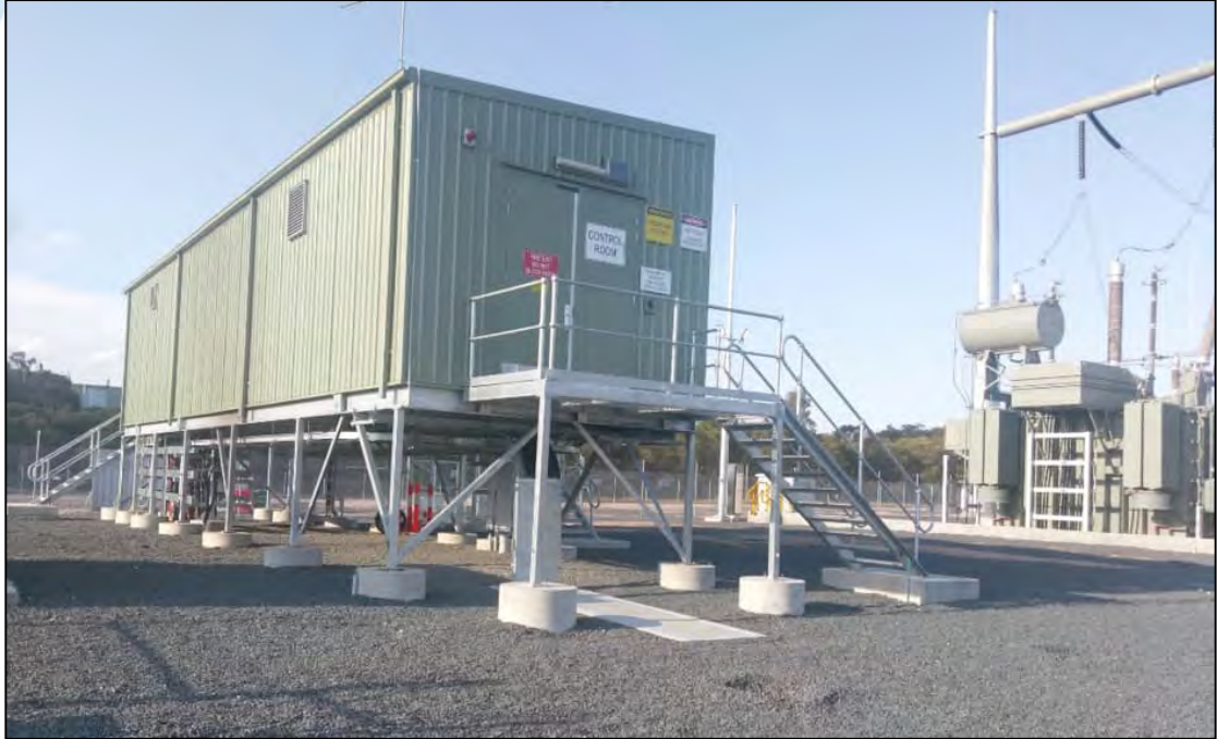
Figure 4-6: Example of a Typical Switch Room
