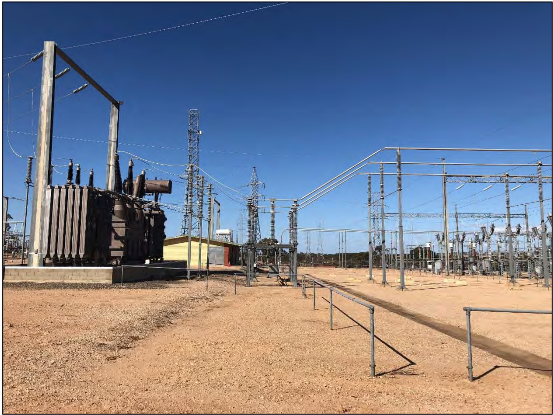
Figure 4-4: Examples of Transmission Substation Infrastructure
