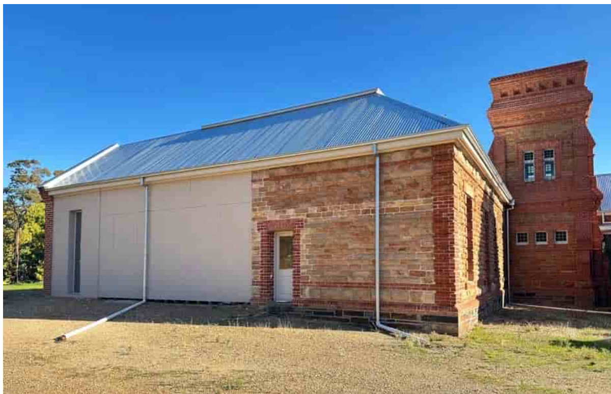
Figure 10: Eastern view of the south wing and tower, 2025 Source: Hosking Willis Architecture
