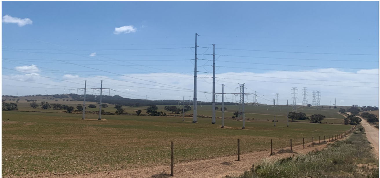
Figure 8:: Existing electricity transmission infrastructure – photo taken 23 October 2024
