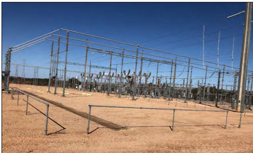
Figure 12e: Example substation
