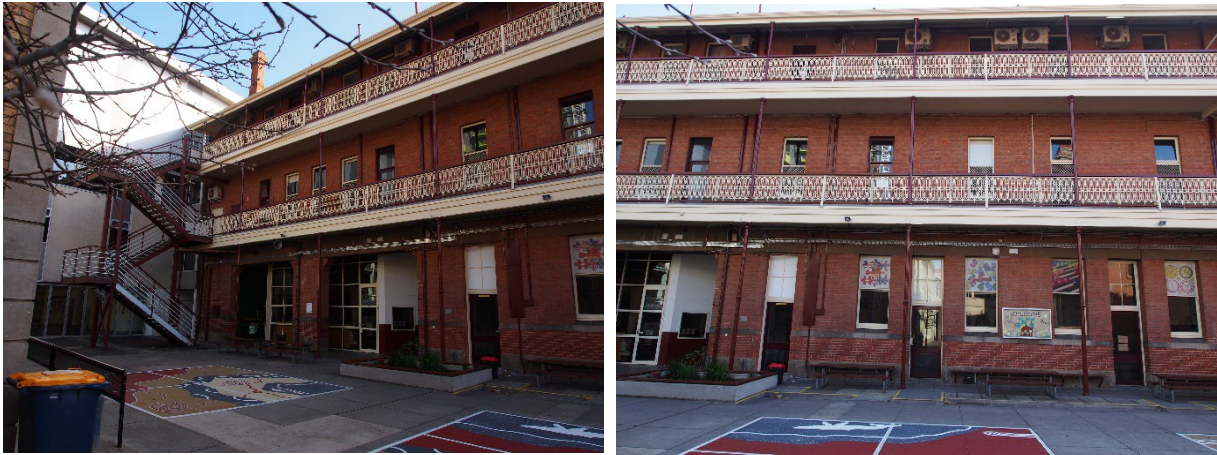
Figure 09 and 10: Dunlevie Building external views of southern wall showing external balconies and external stair
