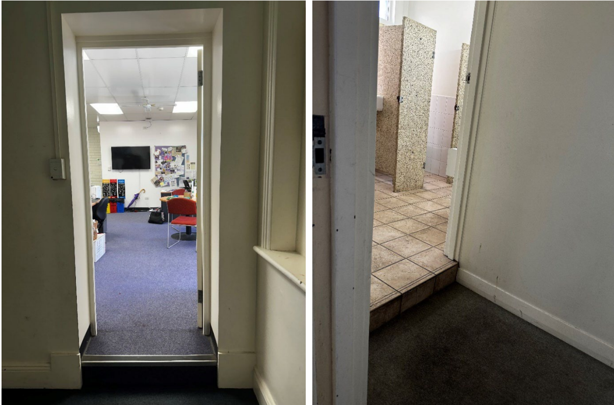
Figure 17 and 18: Dunlevie Building view step hazards to classroom and amenity environments
