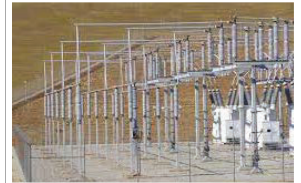
EXAMPLE BUS PIPES, 6-10m IN HEIGHT
