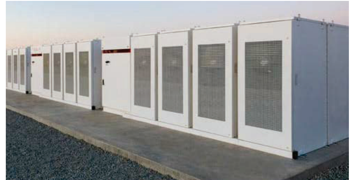
EXAMPLE BATTERY, HORNSDALE POWER RESERVE, SA
