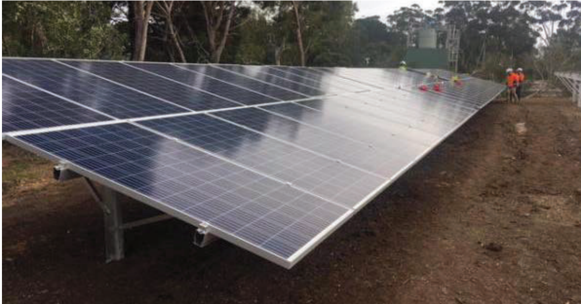
EXAMPLE GROUND-MOUNTED SOLAR ARRAY PROVIDED BY GREEN GOLD ENERGY
