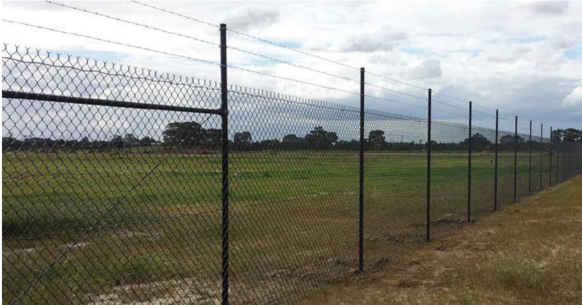
2.3 METRE HIGH SECURITY FENCE
