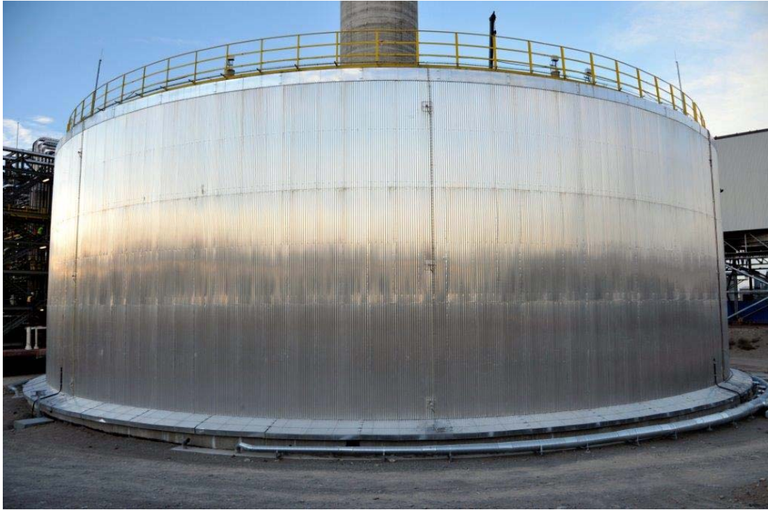
Figure 2-6 Molten salt storage tank
